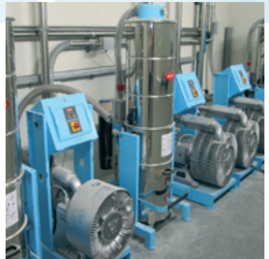
Side channel pumps battery.
